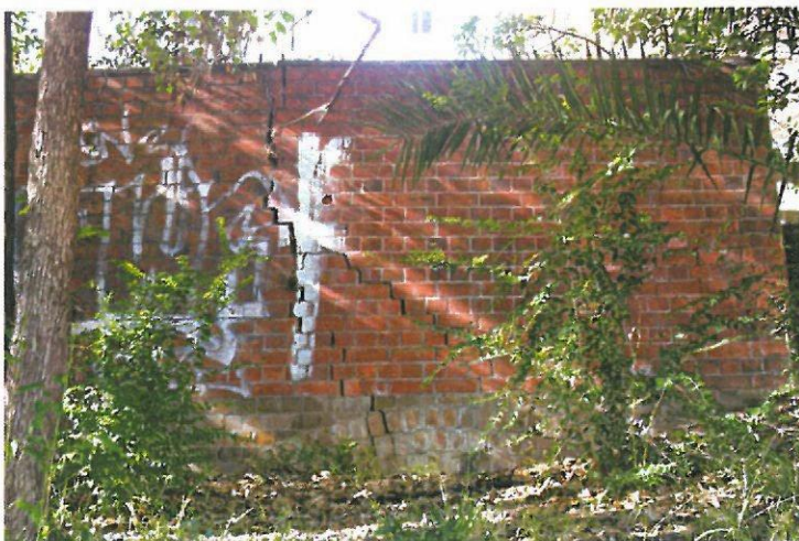
Plate 3 - view of damaged brick wall within railway corridor adjacent to railway platform
